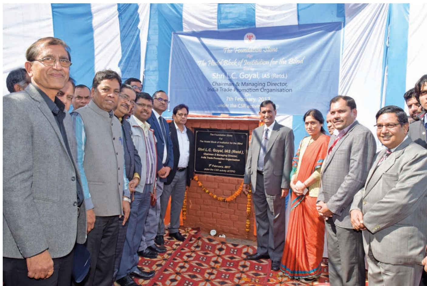
Shri L.C. Goyal, CMD, ITPO laying foundation stone for construction of Hostel block of the Institution for blinds at Panchkuian Road, New Delhi under the CSR initiatives along-with ED, ITPO and other senior officials.
